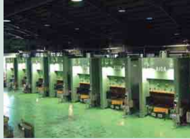
FPD Back Cover Manufacturing Facility
