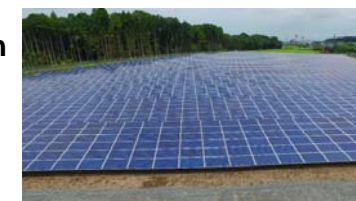
Haru Mito Solar Power Generation
