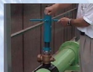
3. Drill a hole in the pipe (the water service is not interrupted).
